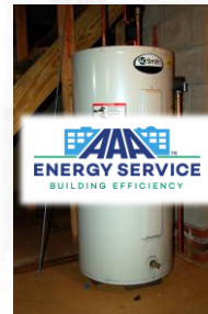
New water heater
